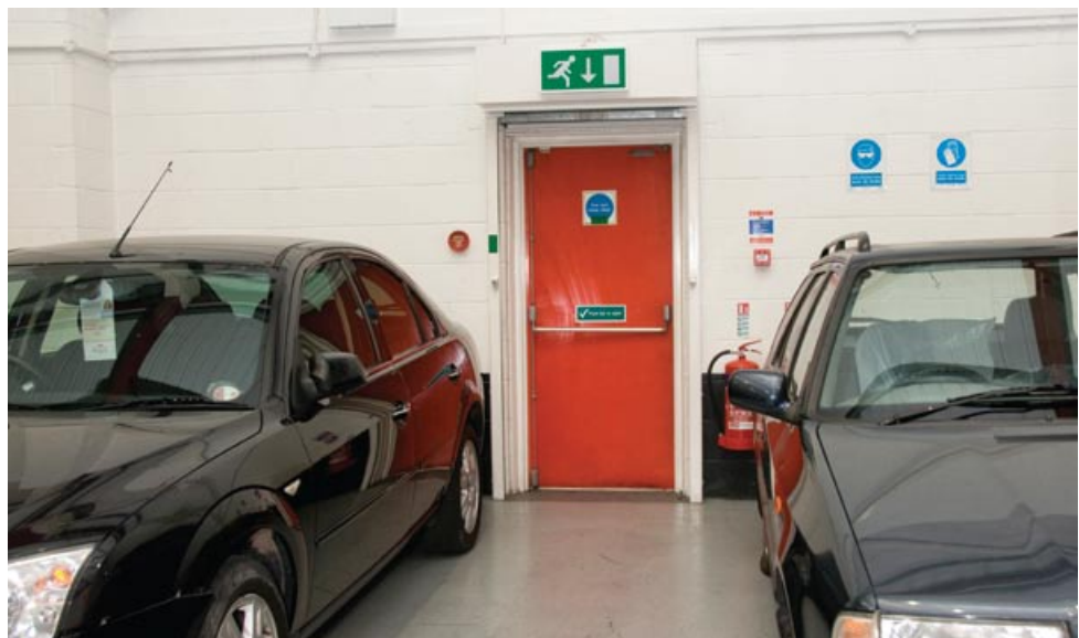
Figure 70 Keep emergency exits well signposted and clear of obstructions
