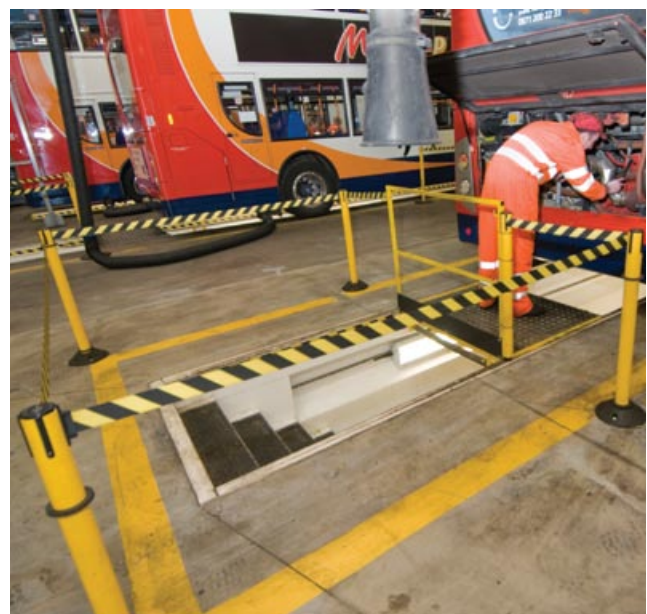
Figure 64 Pit bridge with one handrail removed to provide access to the rear of a bus. Extendible barriers provide a warning about the open area of the pit
