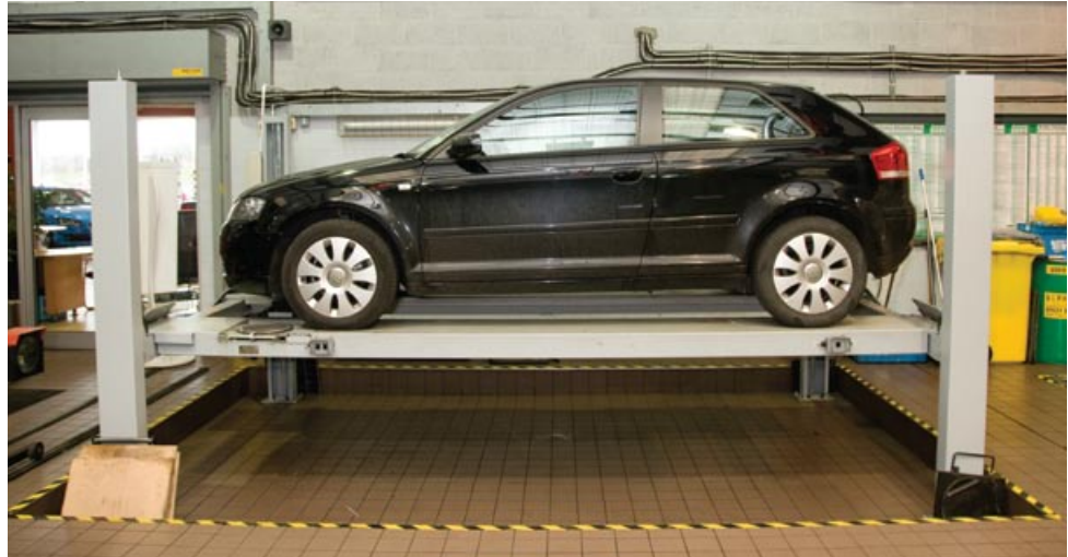
Figure 50 Four-post lift with recessed floor
