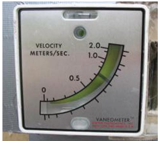
Figure 16 Example of a swinging vane fitted to a spray room
