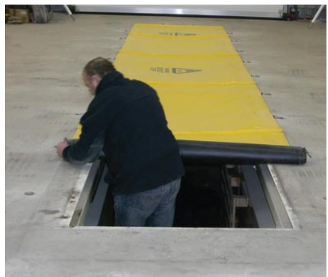
Figure 61 Reinforced fabric cover being fixed in place (photograph courtesy of Everquip Garage Equipment Ltd)
